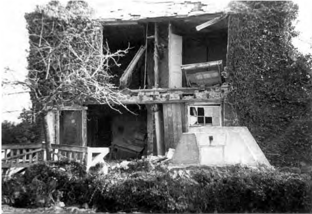
Rear of 100 Honey Lane. Damage to the former Millhouse [Carter]
